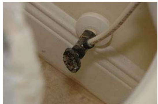
Corroded shut off valve
