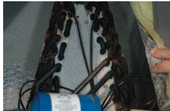
Sulfide corroded coil
