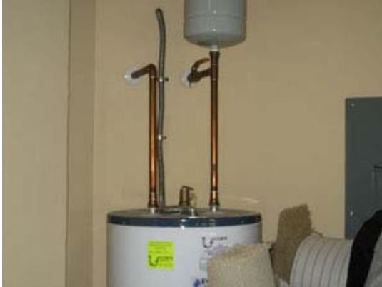
Normal copper plumbing
