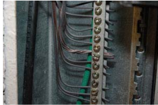
Black corrosion on wiring
