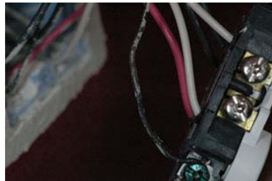
Black corrosion on wiring
