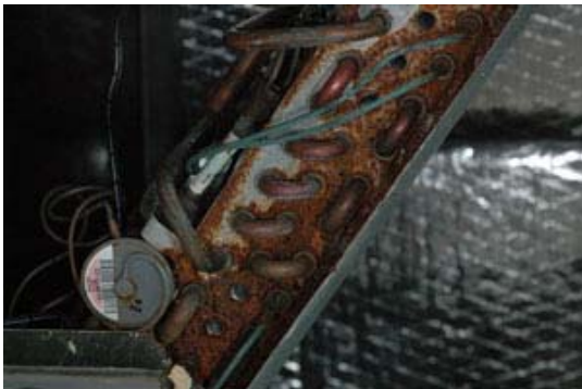
Normal copper in a rusty steel frame
