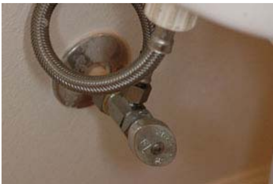
Normal shut off valve
